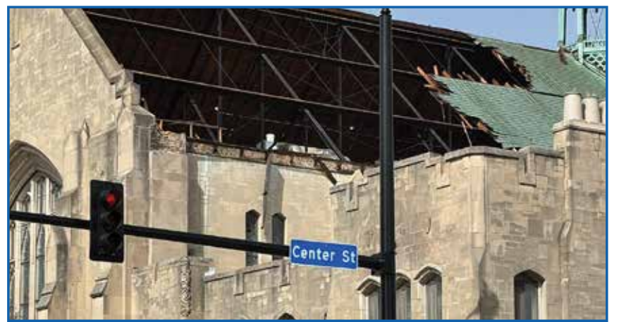
Most of the east side of the sanctuary roof blew off and much of the debris landed on Center Street.
