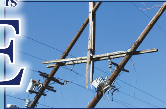
Posts and power lines remain damaged following Hurricane Maria. Authorities have announced that restoration of power could take more than six months. Photo by the Rev. Gustavo Vasquez, UMNS.
