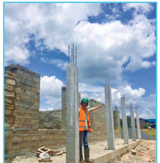
Rev. Young Son (Christina) Kim stands between columns that will frame the science labs at the Global Mission Secondary School in Tanzania currently in its 2nd phase of construction.
