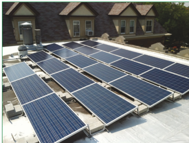
Euclid Avenue United Methodist Church in Oak Park, installed a rooftop solar power system in 2014 to generate and supply electricity to its building.
