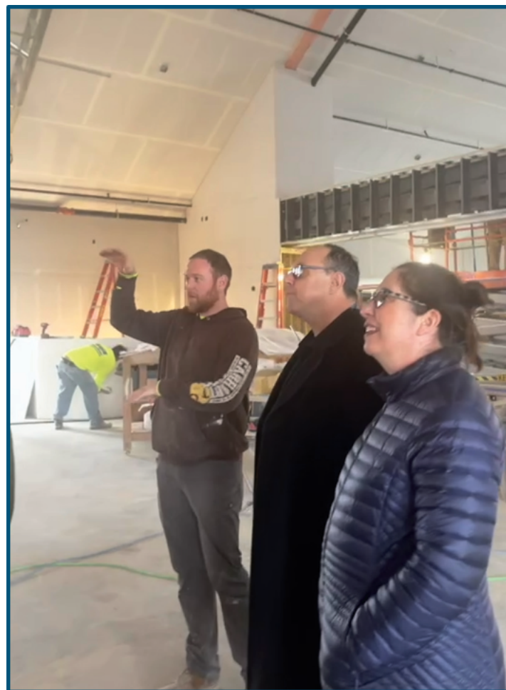
Shaun Chapman, Project Manager for Irving Construction, explains the progress at the First UMC in Dekalb, IL construction site to Bishop and Julie Schwerin.
